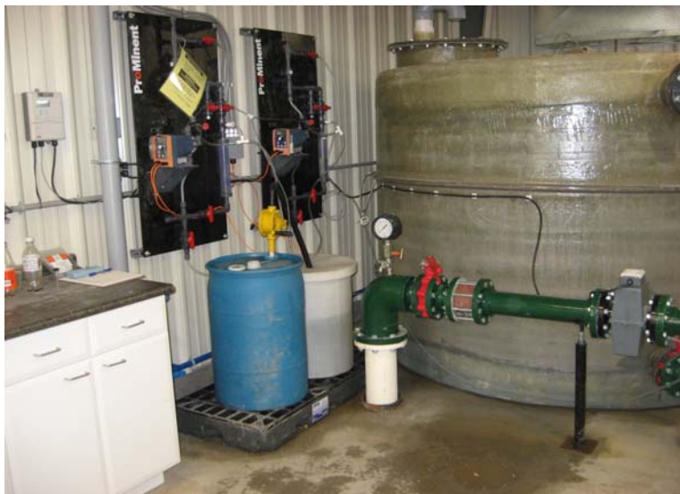
Figure 8. Inlet from well, flow meter and chlorine dosing equipment. (Note lab bench and equipment at left.)
