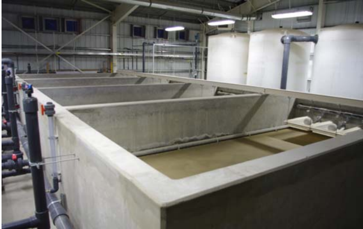
Figure 13. Interior view of water treatment plant.
