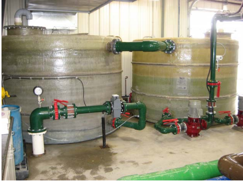
Figure 9. Two contact tanks used to ensure formation of micro-flocs and transfer pumps that take the water to the filters.
