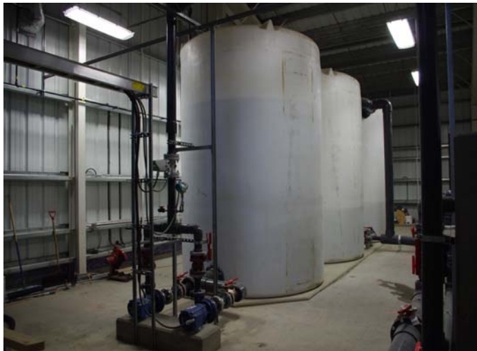
Figure 14. Contact tanks and transfer pumps.
